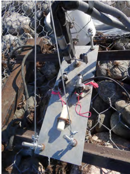
Figure 44: Metal frame for installation of OBS, diver and conductivity sensor
