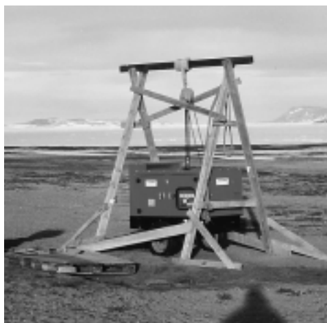
Fig. 2.1. A new 14.4 kW generator was purchased in 1999. The generator weighs 600 kg, and a crane was necessary to unload the generator from the Twin Otter. Photo: Aka Lyngø, PolarPhotos.
